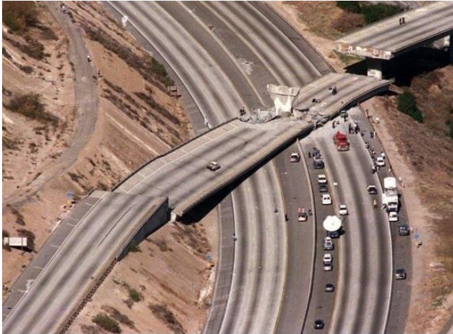
Bypass falls on freeway during the 1994 Northridge Earthquake making it impossible to transport relief aid until removal and inspection for safety.
